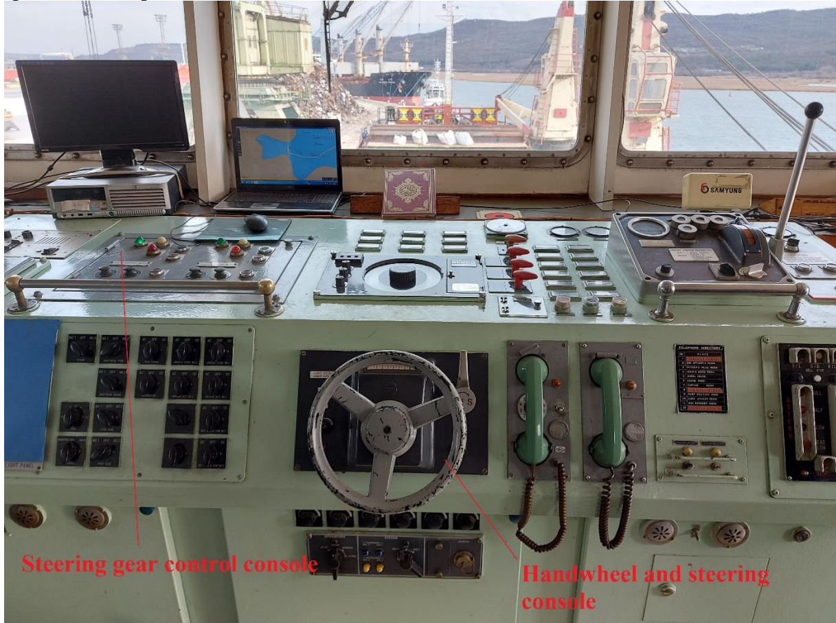
Figure 4 – Ship's bridge with the steering gear console and handwheel and steering console
