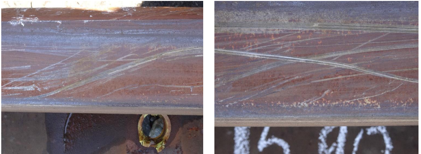
i. j. Fig. 50. Surface of the head of the left tongue of switch № 20 between the 4th and 6th meter
